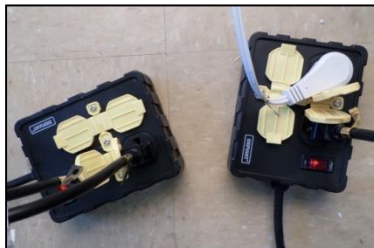
Figure 2.3: Breaker Boxes with Power Cords Plugged-In
